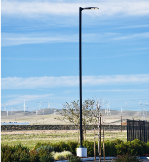
Typical Single-Head Parking Lot Lighting
